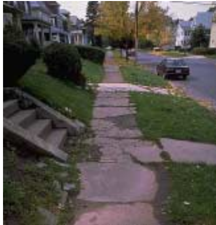
Inadequate maintenance of sidewalks makes a short walk difficult to maneuver.
