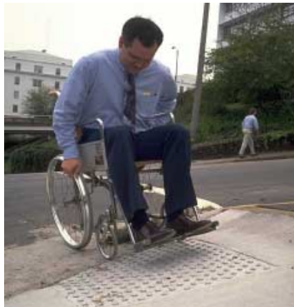
A pavement grinding project left an exaggerated lip at this curb cut.
