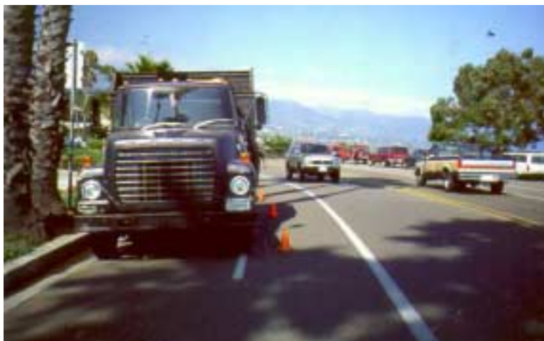
Utility work in bike lanes can often be accomplished without blocking the entire lane.
